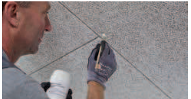
If coloured screws are not used, paint over the screw heads with the paint supplied or a suitable equivalent using a fine brush and suitable amount of paint. Screw heads must be flush with the tile surface.
